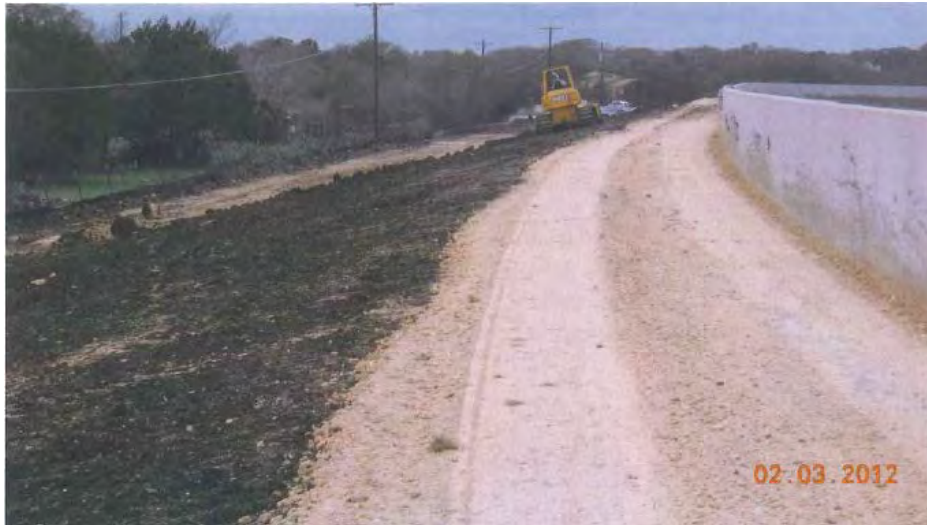
Repair of slope failure caused by Tropical Storm Hermine at Dam 13A
