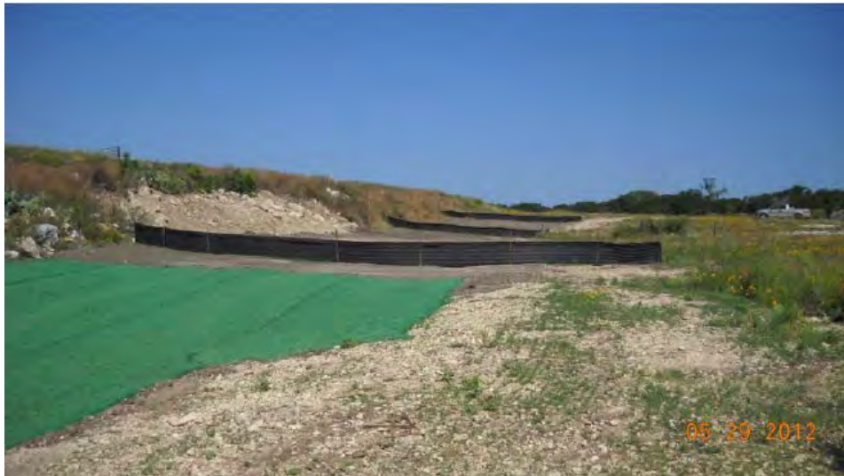
Repair of Erosion caused by Tropical Storm Hermine at Dam 6 Auxiliary Spillway
