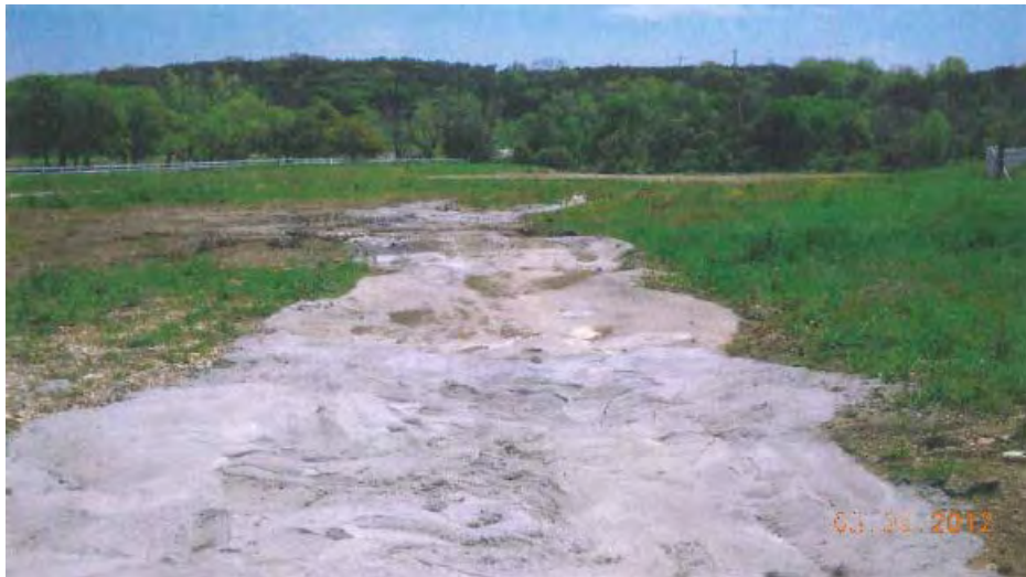
Repair of Erosion caused by Tropical Storm Hermine at Dam 4 Auxiliary Spillway
