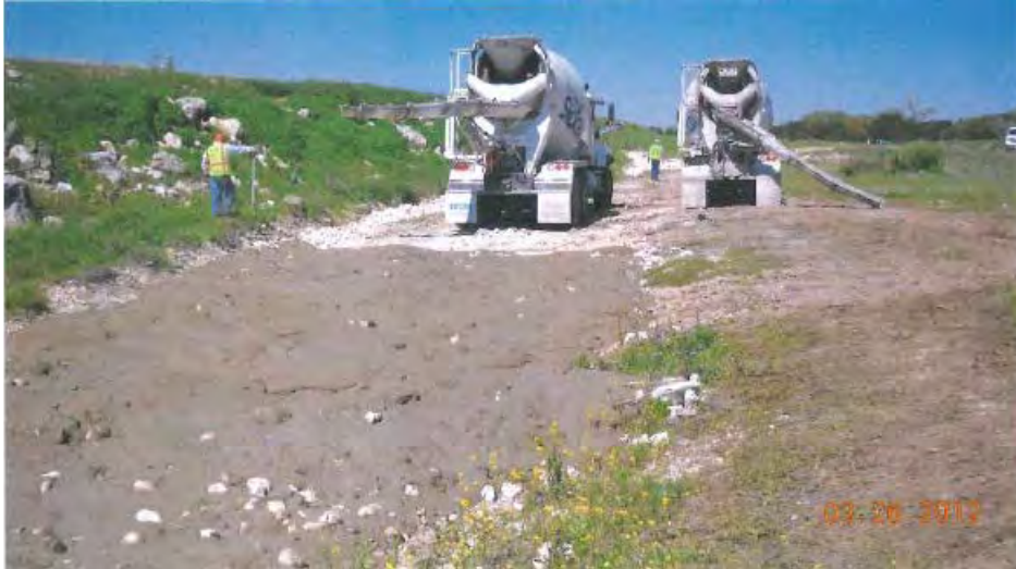
Repair of Erosion caused by Tropical Storm Hermine at Dam 6 Auxiliary Spillway
