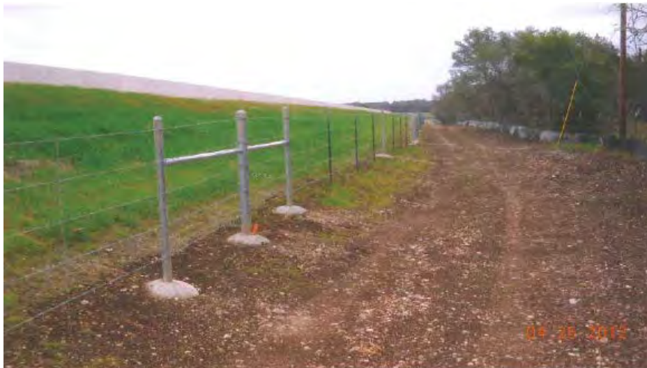
Repair of slope failure caused by Tropical Storm Hermine at Dam 13A
